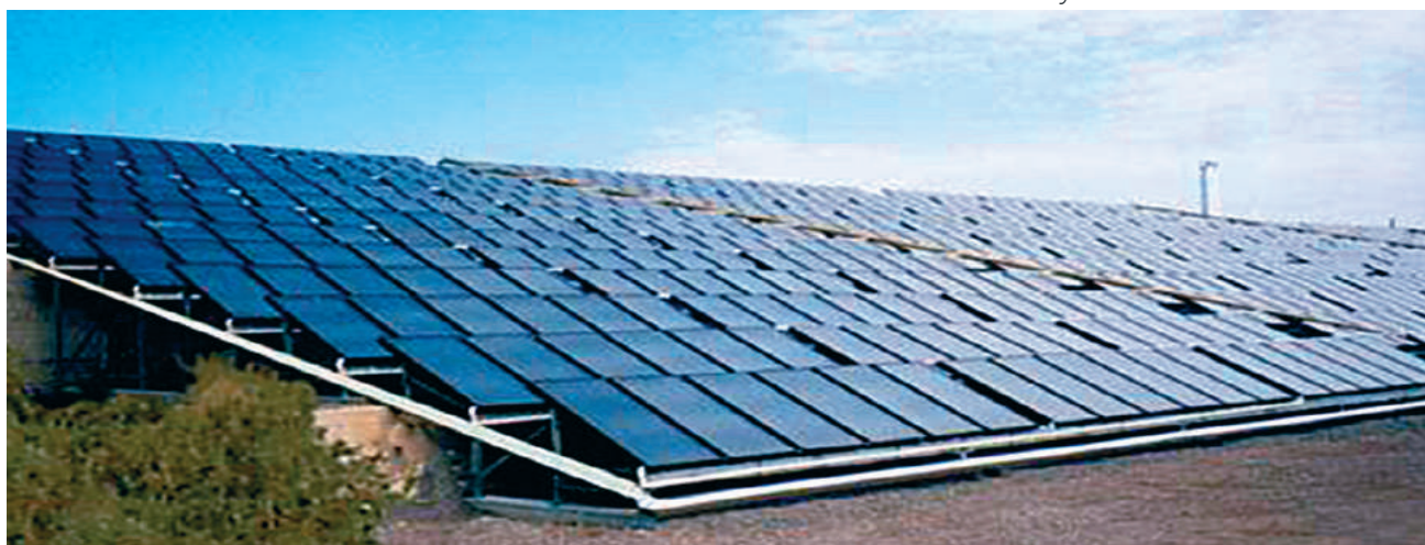
SARANTISS.A., 1999-Solar Air -Conditioning 700kw
