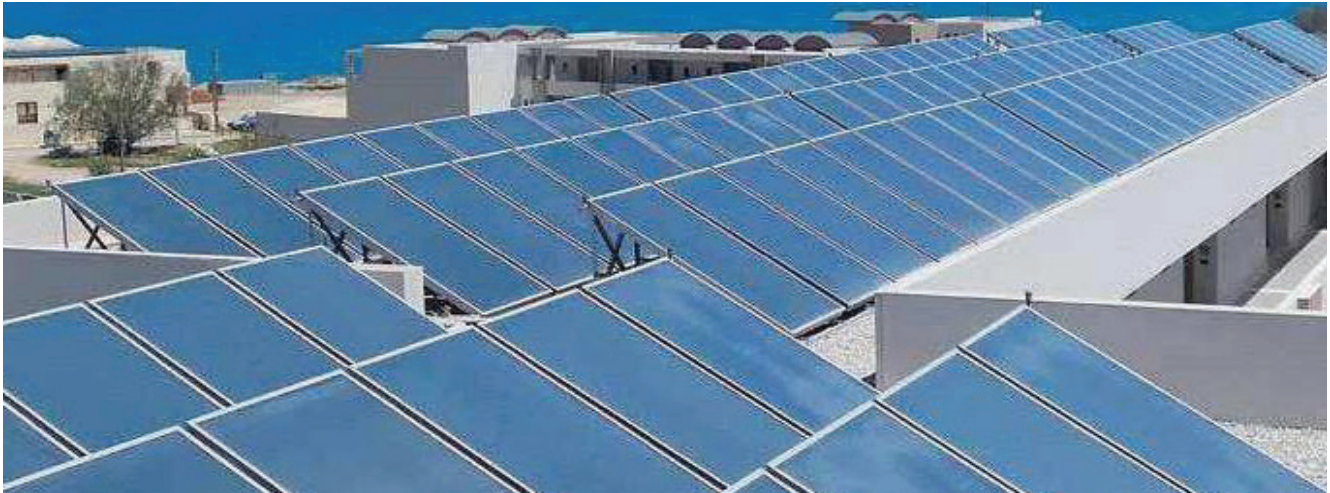
KOLYMBARI BEACH HOTEL, 2010 - CHANIA, CRETE / SANITARY HOT WATER
