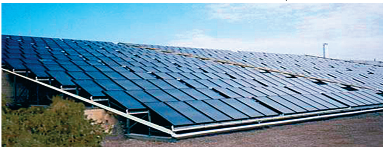
SARANTISS.A., 1999-Solar Air -Conditioning 700kw
